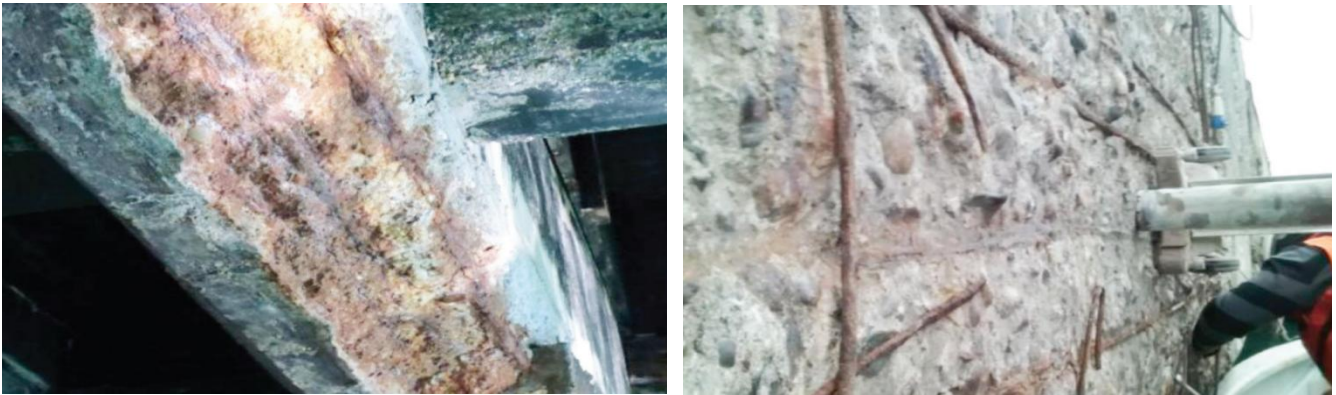
Figure 1. Deterioration due to corrosion effect on port structures.
