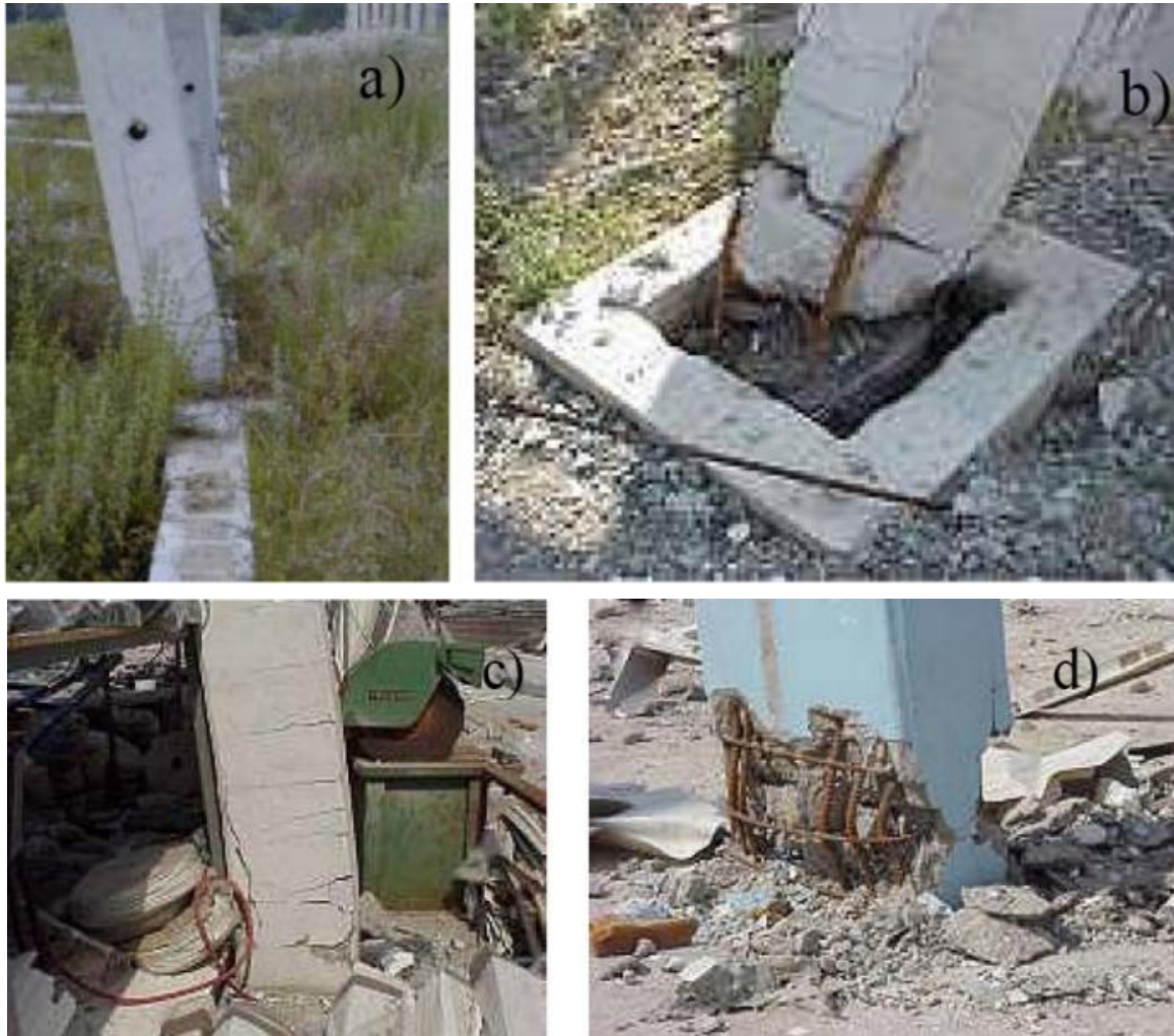
Figure 1. Seismic damage patterns present in precast industrial reinforced concrete columns in Turkey; a) Concentrated flexural patella damage in column base (Posada and Wood, 2002), b) Concentrated damage in column base with plinth type foundation, c) Flexural patella damage distributed over 800 mm of column height and d) Severe concentrated flexural buckling damage at column base (Saatcioglu et al., 2001).
