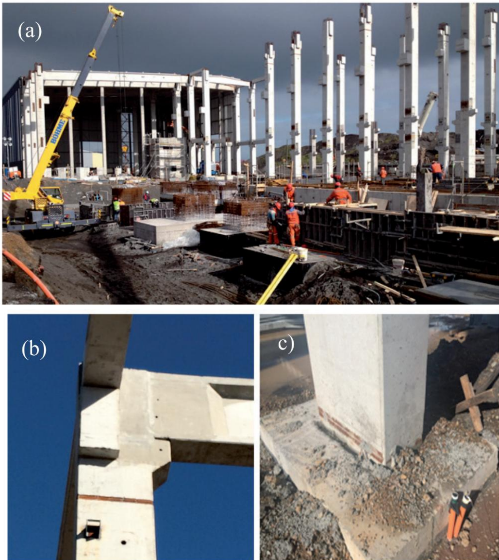
Figure 5. (a) Construction and assembly of structural elements, (b) Hybrid connection at top and (c) Bottom edge of a column.
