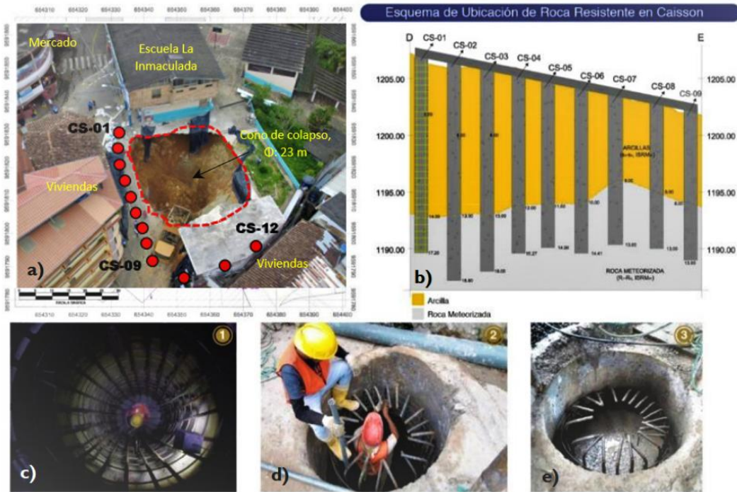
Figure 3. a) Spatial distribution of the caisson piles. b) Profile with the location of the piles in soft rock (16.76 MPa). c and d) upward iron reinforcement process. e) 280 kg/cm 2 concrete curing process.
