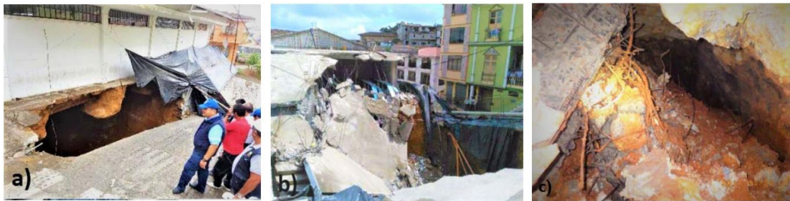
Figure 2. a) Beginning of collapse with a 10 m cone. b) Destabilization of structures. c) Debris (columns, hoses, cables, blocks) inside the gallery that caused the subsidence of the ground at surface.
