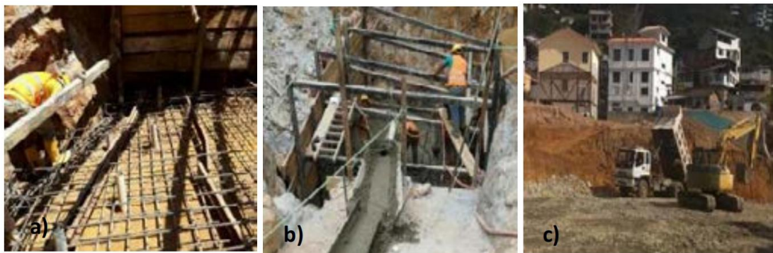
Figure 4. a) Backfill + drains + perimeter beam + iron reinforcement. b) Casting of slab. c) Backfill with compacted material Sub-Base class 3.
