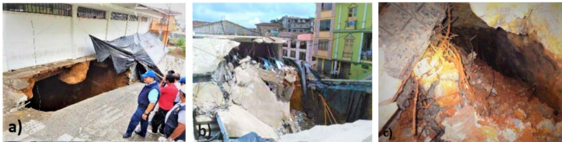
Figure 2. a) Beginning of collapse with a 10 m cone. b) Destabilization of structures. c) Debris (columns, hoses, cables, blocks) inside the gallery that caused the subsidence of the ground at surface.
