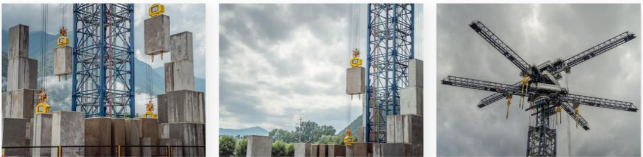
Figure 1. Vault energy gravity pile. Proof of concept executed in Switzerland (Energy Vault, 2022).
