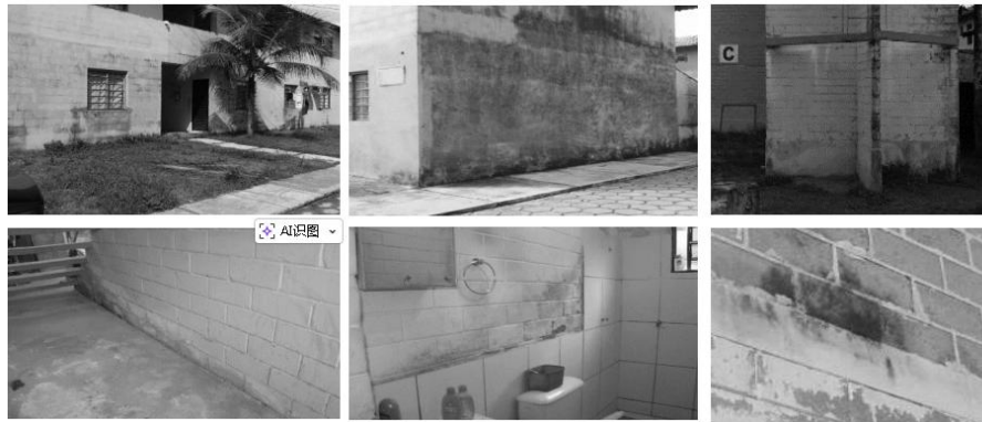
Figure 3: Set of pathological manifestations found in the residential building. Source: the author
