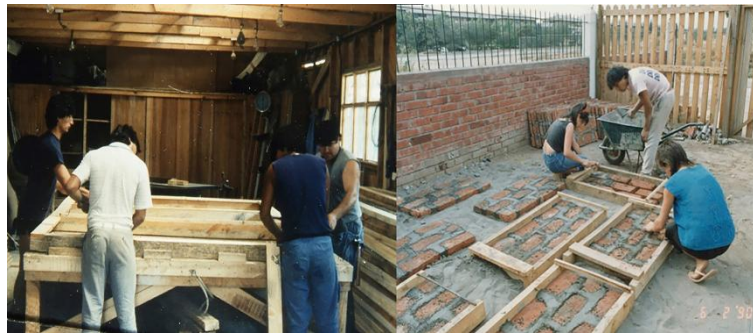
Figure 5. Prefabrication of wooden wall panels in the workshop and prefabrication of brick tiles in the workshop courtyard
