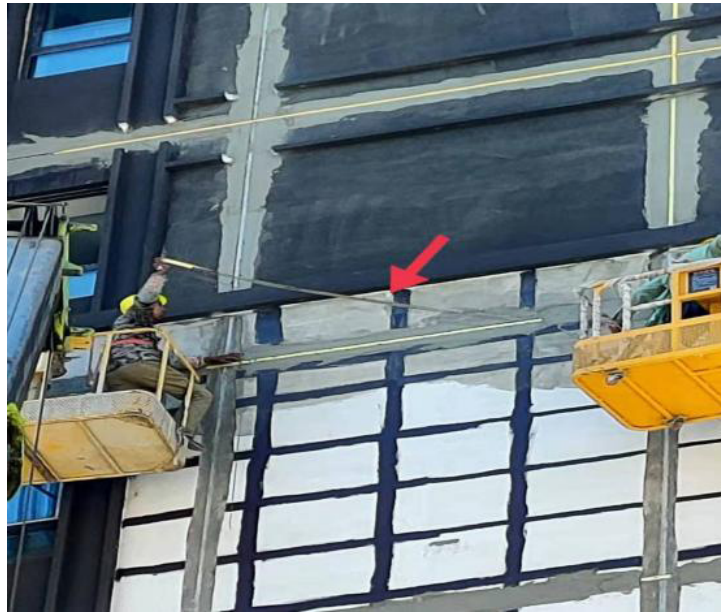
Figure 8. The operation process of the double-layer tape for the partition and joint
