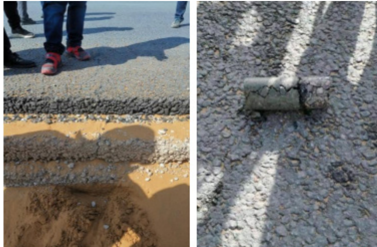
Figure 2. Crack running up to down
