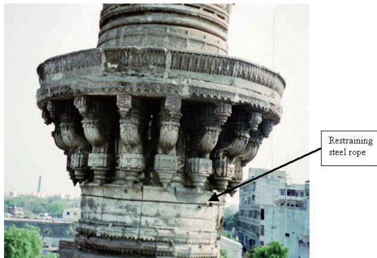
Figure 7. Stainless steel ropes introduced into the courses of cylindrical masonry structures to secure them against lateral failure in Bashir's Minars, Ahmadabad
