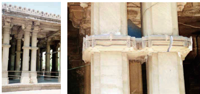
Figure 4. Overview and details of cracks at the tomb of Syed Usman at Usmanpura, Ahmedabad
