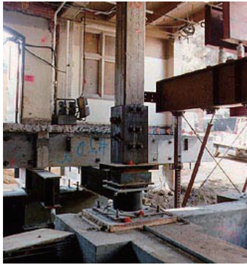
Figure 10. The new base isolator allows the structural support member at the foundation to move horizontally as it absorbs the earthquake forces
