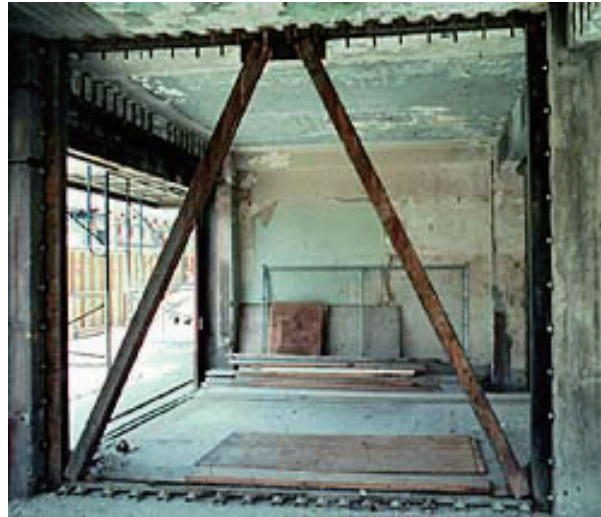
Figure 9. An interior diagonal frame that will dampen and transfer seismic loads in a designed path from foundation to roof
