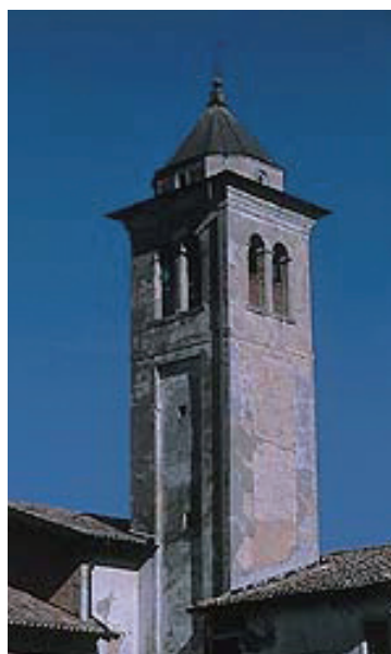
Figure 11. The earthquake-damaged bell-tower of San Giorgio in Trigano, northern Italy, is being restored using a hidden shape-memory alloy device
