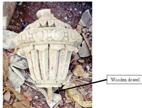
Figure 3. Ornamentation fell from roof level of Amah Vilas, Jamnagar
