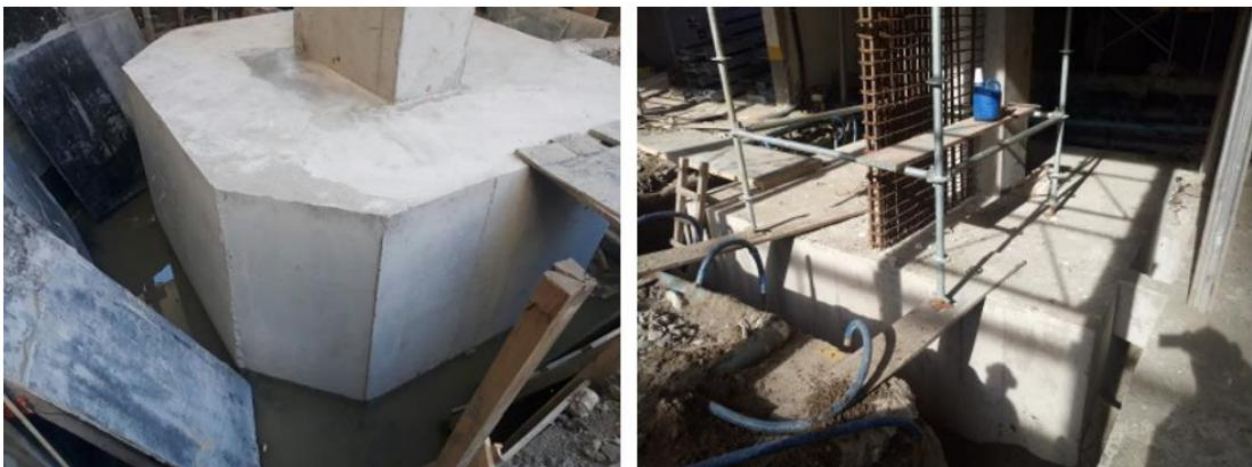
Figure 17. Details of the appearance and surface finish of the reinforced blinding concrete.
