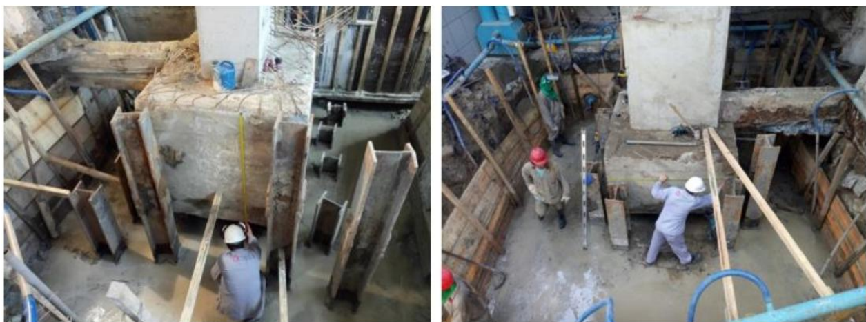
Figure 9. Details of dimensioning of existing pile drivers and metal piles after concrete excavation and construction.
