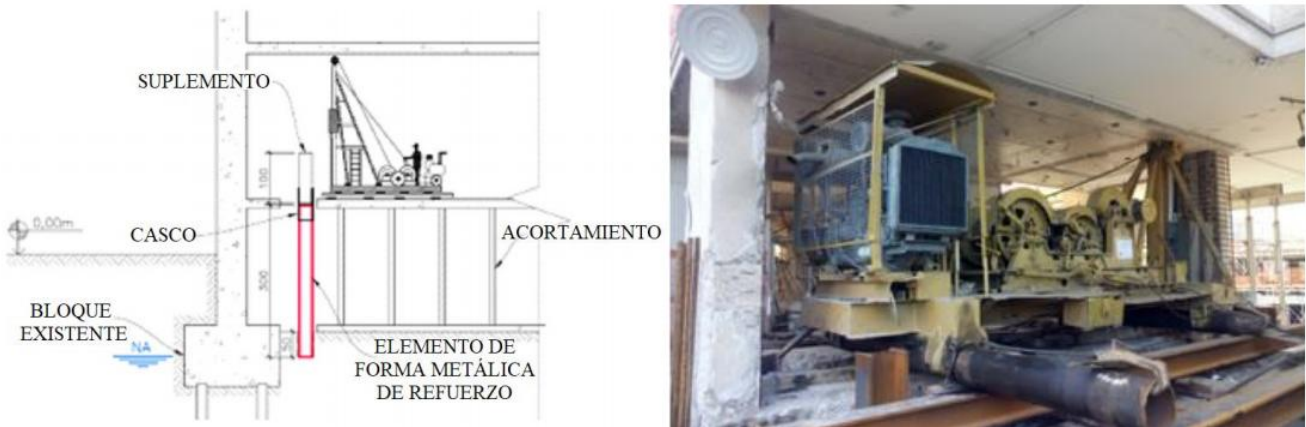
Figure 7. Details of a suitable pile driver positioned between the plates to perform piling services for structural reinforcement piles.
