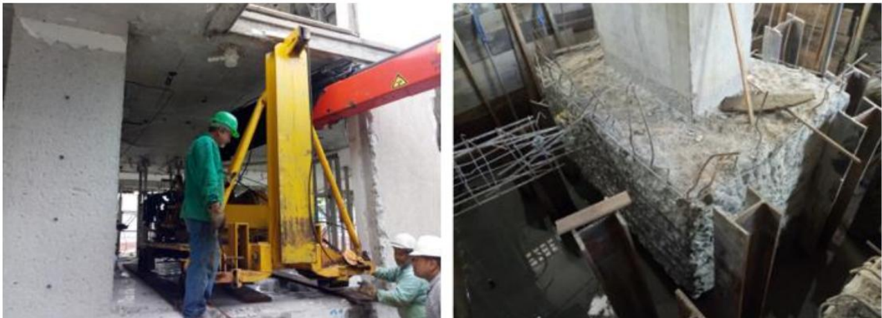
Figure 8. Detail of the execution of the piping works (on the left) and of the metal piles driven around the foundation block to be reinforced (on the right).
