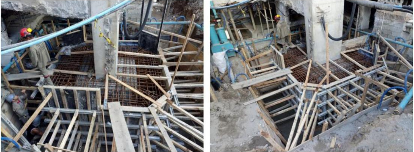
Figure 14. Details of the shapes of the structural reinforcement of the foundation pile caps.
