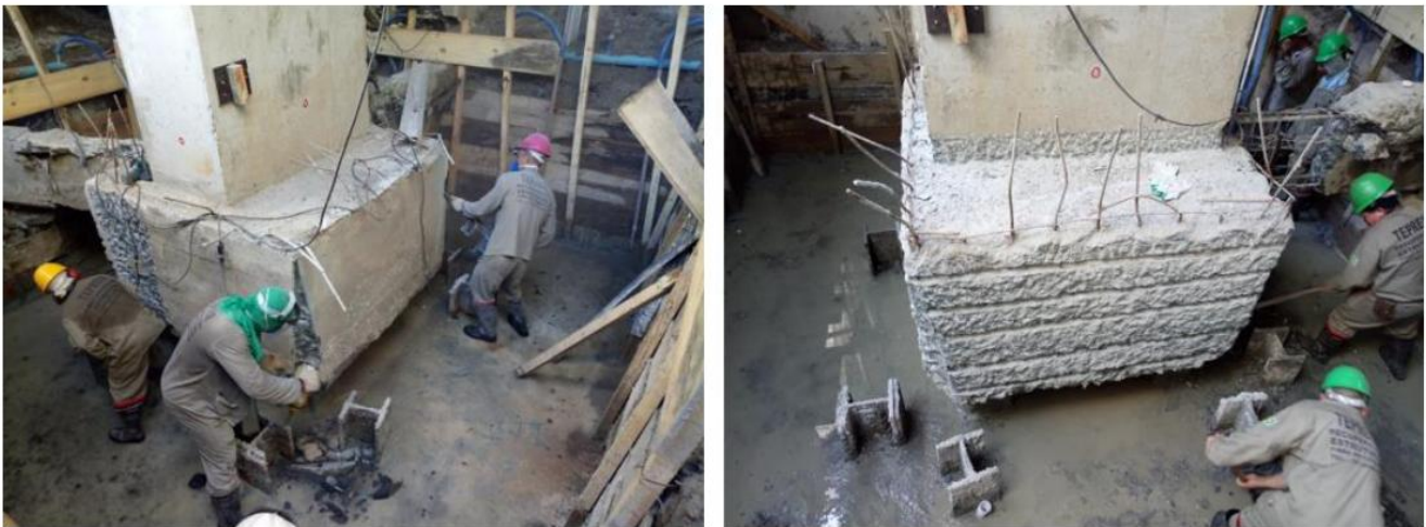
Figure 10. Details of the execution of the chamfers and grooves on the edges and lateral surfaces of the foundation pile caps.
