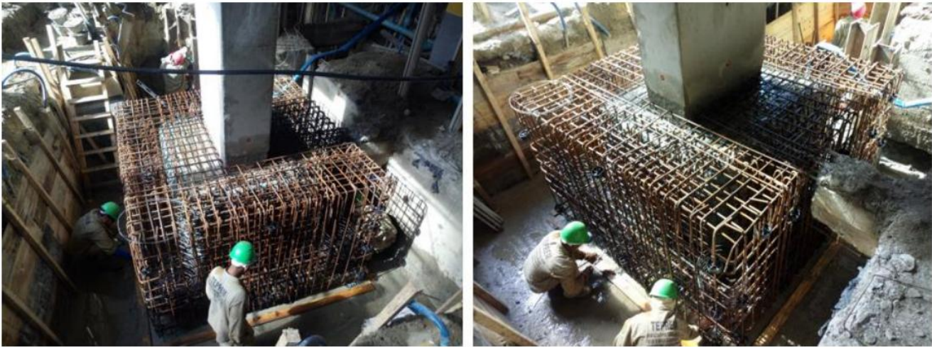
Figure 13. Details of the execution of the reinforcement work of the foundation block.
