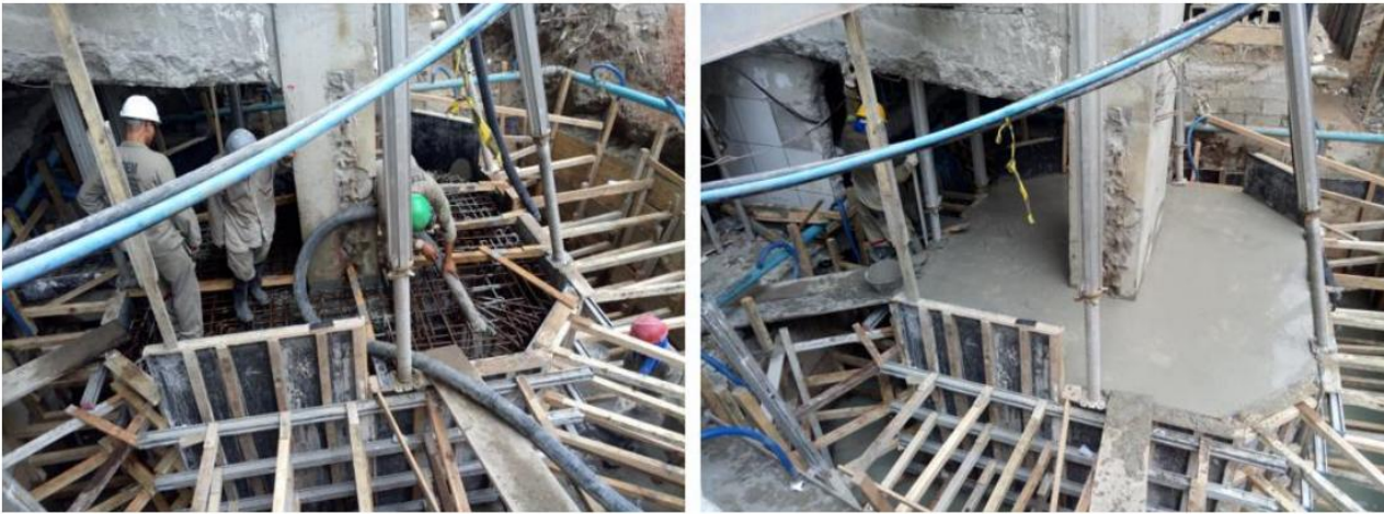
Figure 16. The details of the foundation block reinforcement emptying are made of self compacting concrete.
