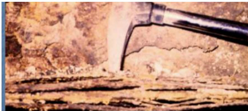
Figure 5. Exfoliation corrosion on water treatment plant.
