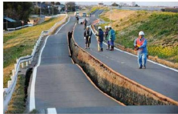
b) Effect of liquefaction on roads.
