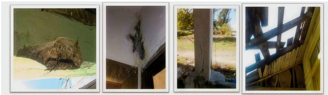
Figure 2. Evidence of the main pathologies found in buildings with construction types I (Concrete), II (Masonry), III (Masonry and Light Roof), and VI (Wood) 2018-2019. (Authors)
