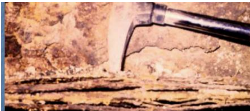
Fig. 5. Exfoliation corrosion on water treatment plant.
