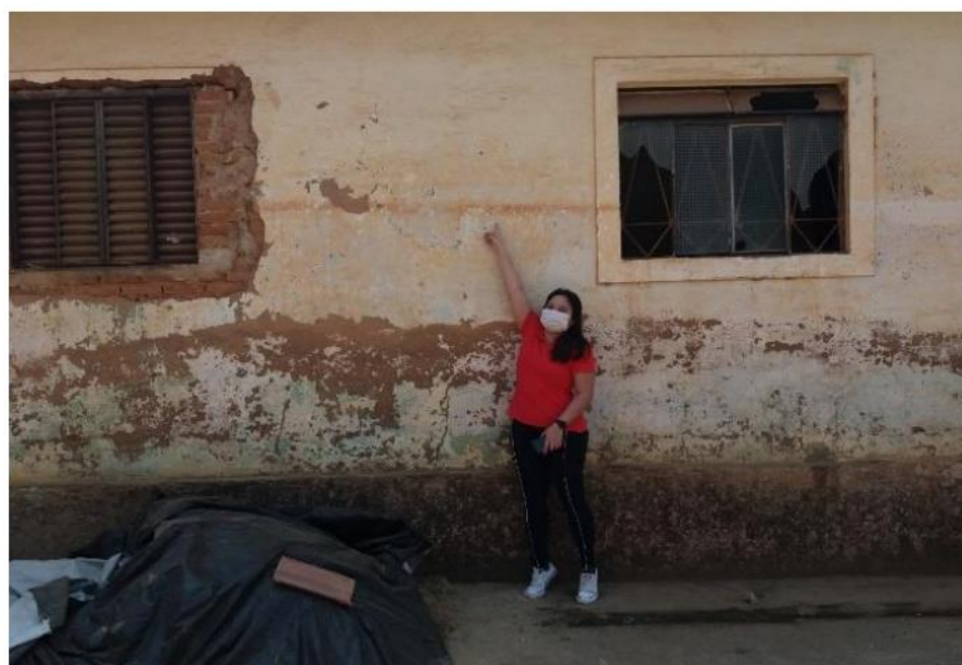
Figure 4. Water level mark reached in the 2000 flood
